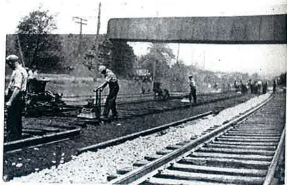
A large rail laying gang of an Eastern road is being served by three Adzing Machines.
