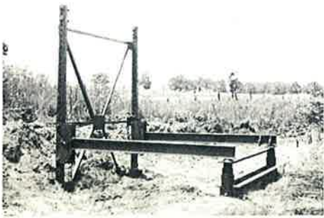
Closeup of Cribex setoff. Note adjustment of back for variable bank contour.
