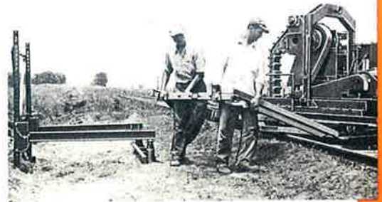
Cribex has been moved from platform to turntable and is being turned 90°.
