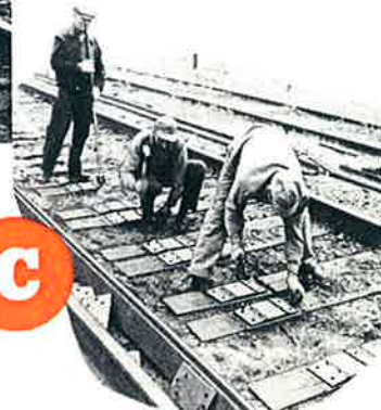
B After the holes have been drilled in the ties, conical shaped wooden pegs, which were distributed when the plates were pre-gaged, are driven into the two holes drilled by the DUN-RITE. The pegs hold the tie plates in accurate gage. The rail is then laid, bolted and spiked.
