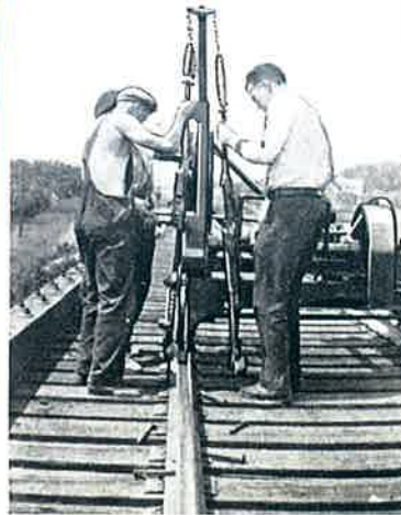
Pulling spikes on a bridge at the rate of 36 spikes per minute.
