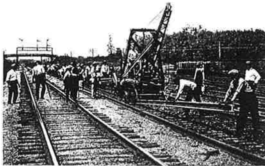
A typical rail laying job for which the Track Machine was used. It is fast enough to keep the large spiking gang busy.
