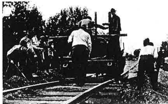
A main line elevation job where the track had to be kept in condition for service. This machine is equipped with run-off wheels.
