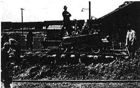
Making a five foot raise in grade, working in soft sticky clay. On the same job the Machine was also used for ballasting.
