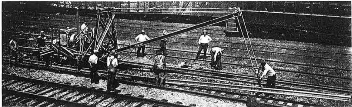
Laying 130 pound, 39 foot rails with the Track Machine equipped with rail laying attachment.
