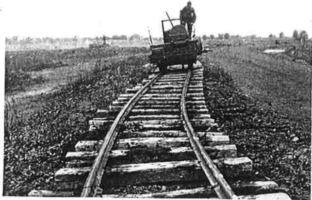
Starting a waste dump for the disposing of the overburden of a clay pit.
