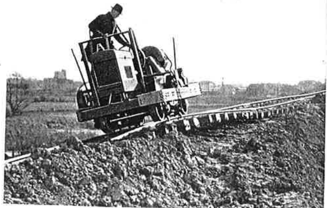
The 36-inch track on this 30-foot fill was raised and shifted by a Nordberg Track Shifter.
